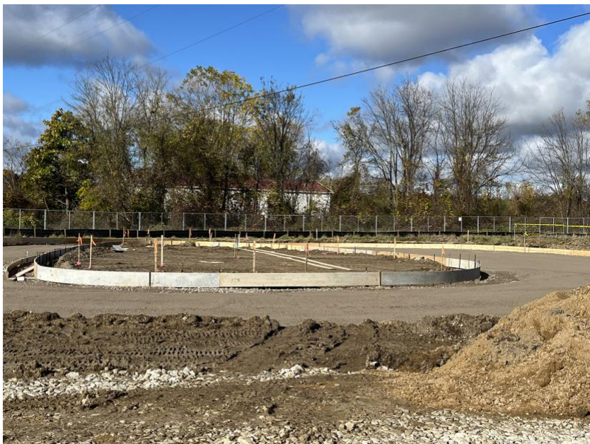
Construction is underway at the future LAFCU Perry ITM/ATM site, located on 2800 W. Lansing Road. The new location will offer 24/7 ATM access and live teller service.
